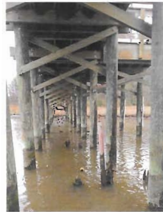
Ghosts from the past: broken pilings from the original Chesapeake Beach Railway peek out in low-tide under the current Rail Trail bridge
